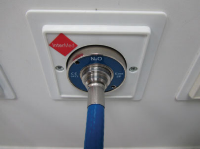
Figure 5.12 Blue tubing into outlet valve.
